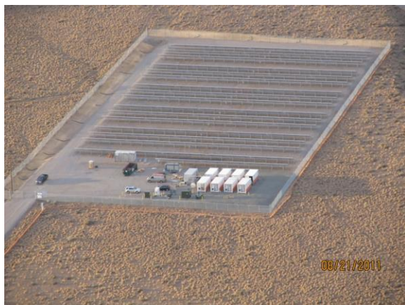
Figure 7 - PNM Prosperity Energy Storage Project - Aerial View
