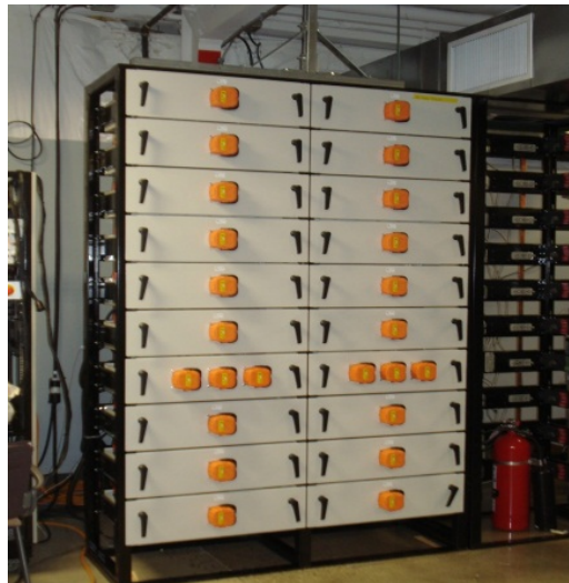
Figure 16.6. One of 20 Modular Battery System Racks at the Salem Smart Power Center 4
