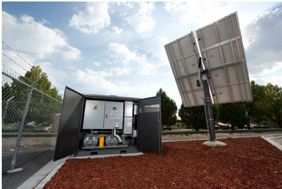
Figure 11.22. Idaho Falls Power Battery Storage and PV Array
