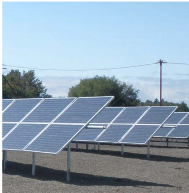
Figure 9.4. Arrays of Standard Polycrystalline PV Panels at the Ellensburg Renewable Energy Park (City of Ellensburg 2013a)
