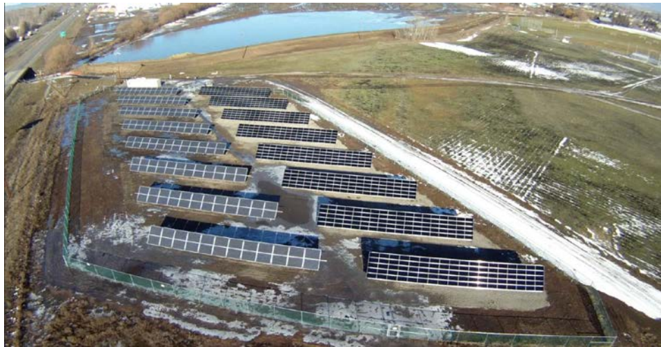
Figure 9.1. Polycrystalline (left) and Thin-Film (right) Solar Panel Arrays at the City of Ellensburg Renewable Energy Park, Ellensburg, Washington 1
