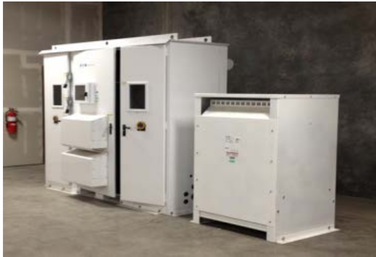
Figure 16.7. Eaton Inverters and Isolation Transformer at the Salem Smart Power Center 1
