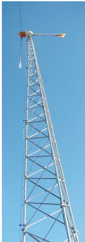
Figure 9.30. 10 kW Bergey Wind System at the Ellensburg Renewable Energy Park (City of Ellensburg 2013a)
