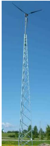
Figure 9.43. 10 kW Ventera Wind System at the Ellensburg Renewable Energy Park (City of Ellensburg 2013a)
