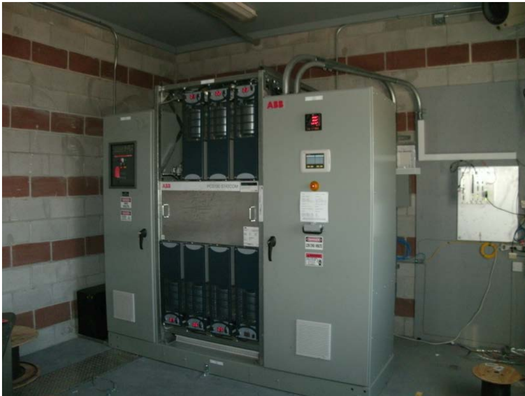
Figure 12.33. 300 kVAr SVC at the Bondurant, Wyoming, Site
