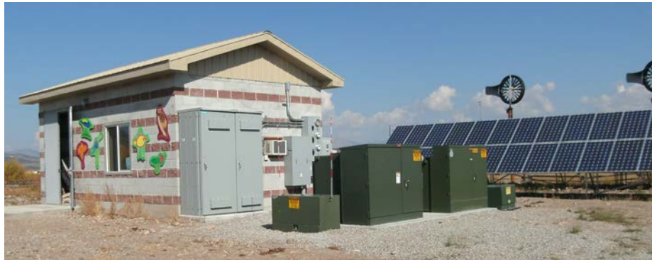
Figure 12.3. Bondurant Site where SVC, Solar PV, Wind, and Battery Systems Resided
