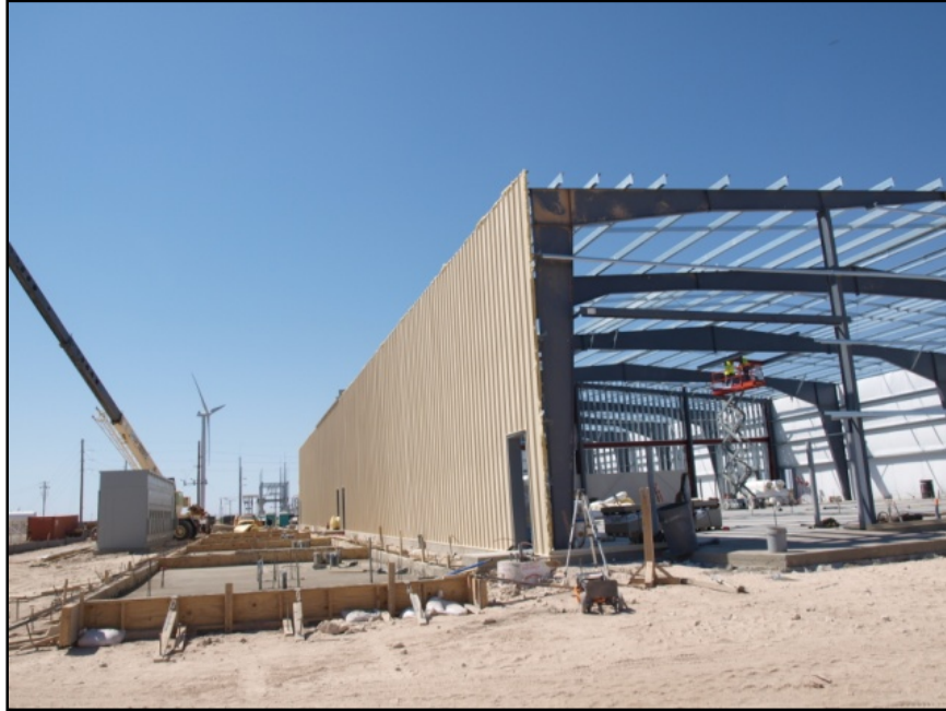
Figure 6-8 East side and unfinished north end of project building (view northeast to south)
