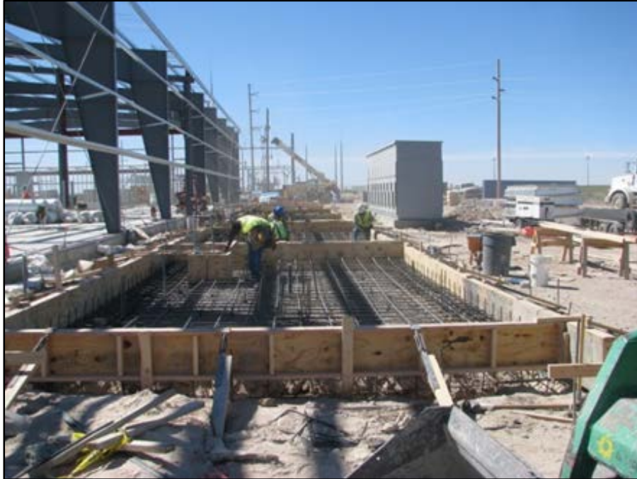
Figure 6-6 Preparations for pouring concrete on the opposite (west) side of the building (view northwest to south)
