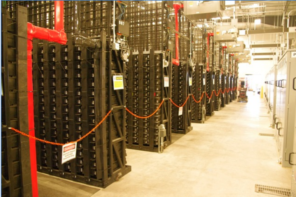
Figure 2-5 PowerCell Modules Installed at Duke Notrees Wind Storage Project (batteries at left, PCSs at right)
