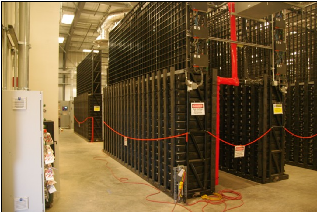
Figure 6-11 PowerCell Modules are arranged in two parallel rows that run the length of the building (one row in foreground, the other row visible at left background).
