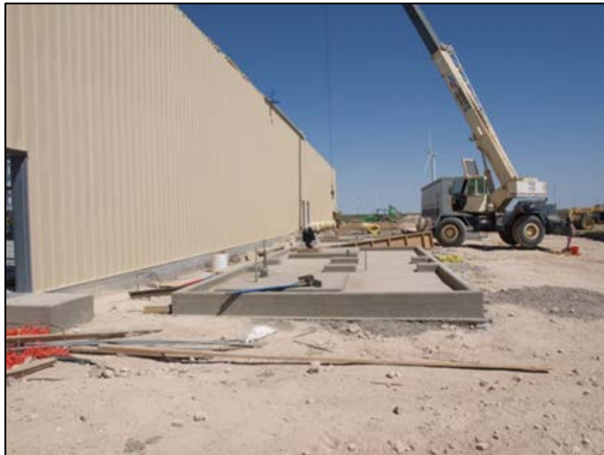
Figure 6-7 East side of building, with concrete pads for transformers in place (view southeast to north)
