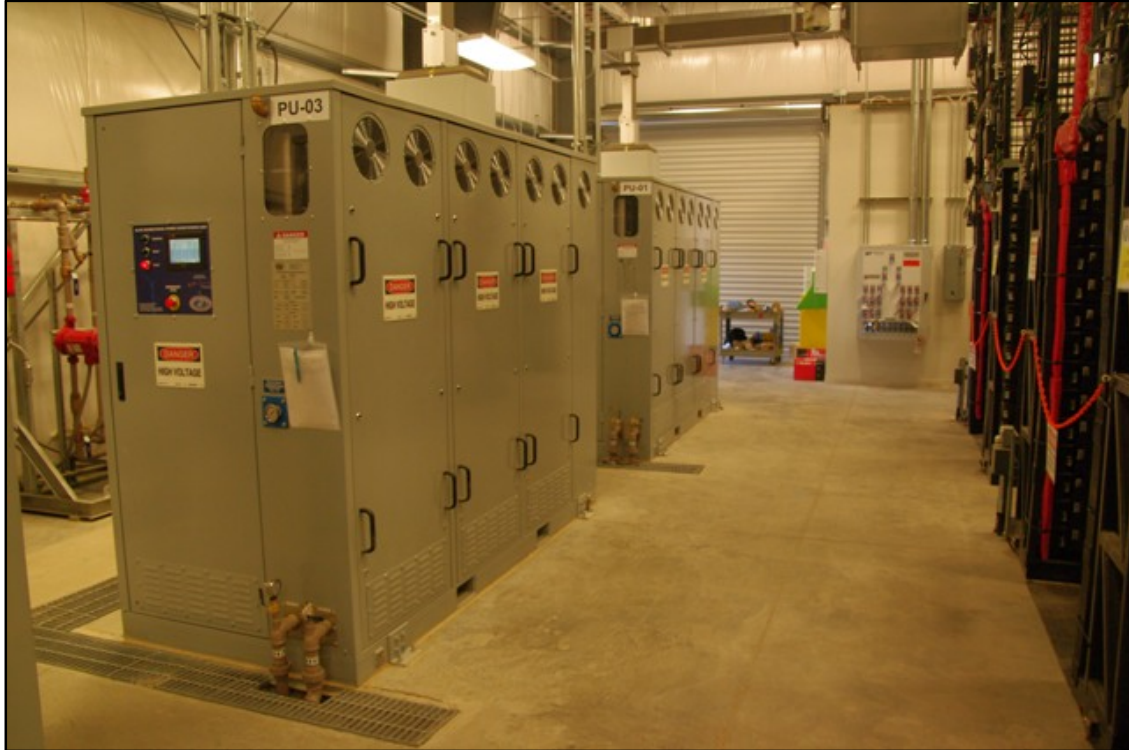
Figure 6-12 Two of the PowerCell Module PCS units (batteries at right)
