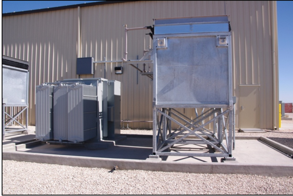
Figure 6-10 Typical transformer (left) with cooling units (right) outside the building
