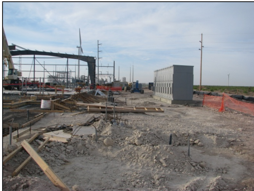
Figure 6-3 Building construction at left, switchgear enclosure at right (view northwest to south)
