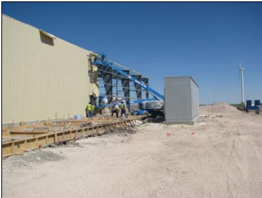
Figure 6-5 Walls along the east side of the building, with concrete forms for transformer pads in foreground and switchgear at center right (view south to north).
