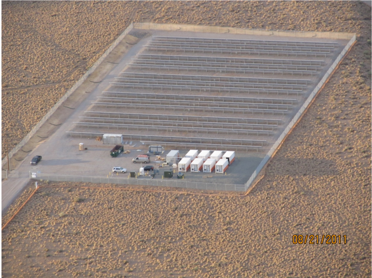
Figure 7 - PNM Prosperity Energy Storage Project - Aerial View
