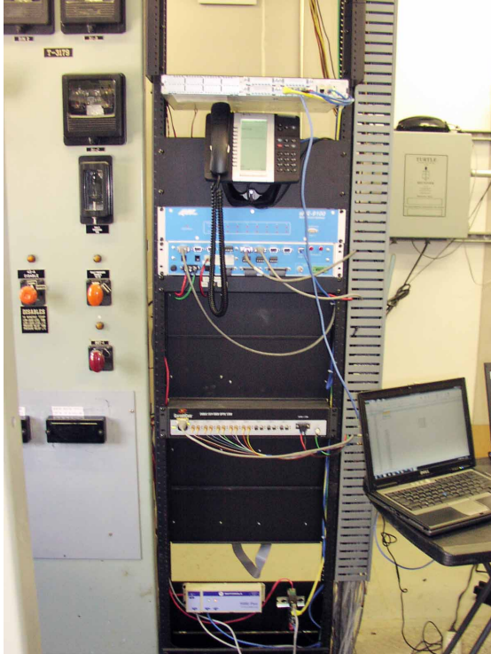
Figure 3: Decker Substation 5 with SGIG Router (above telephone) - QEI RTU (blue)
