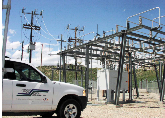
Figure 1: A Remote Powder River Substation
