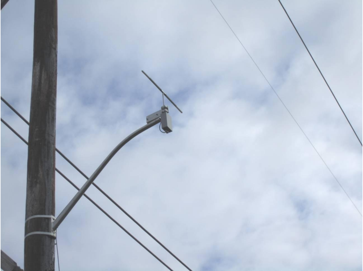
Figure 4-8 ThermalRate Sensor installed
