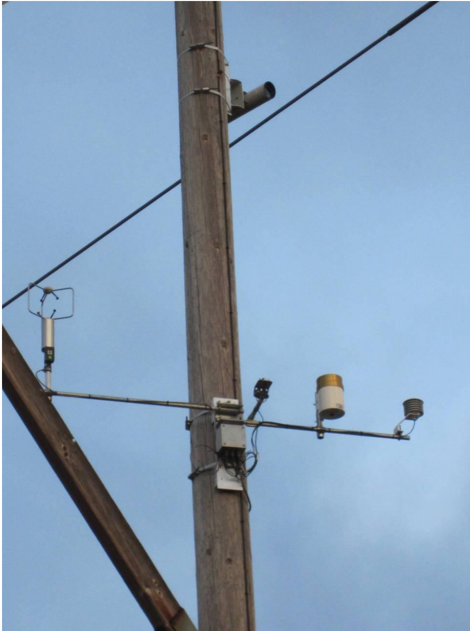
Figure 4-64 Sagometer camera and weather instruments installed
