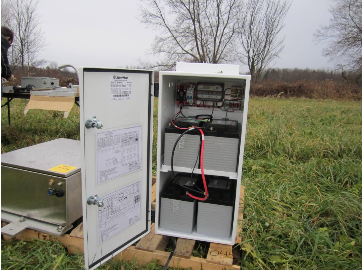
Figure 4-45 ThermalRate battery box
