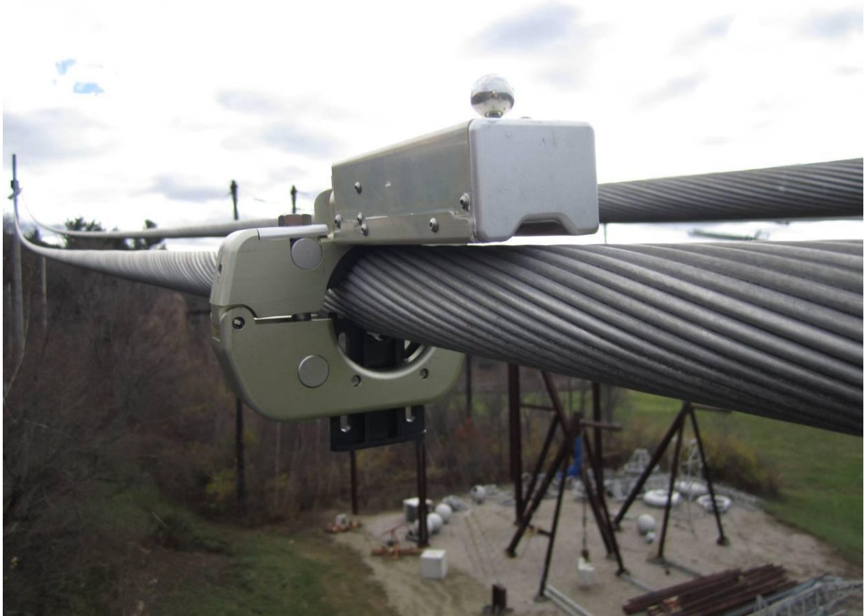
Figure 4-5 EPRI sensor attached to conductor
