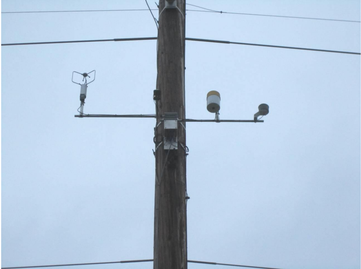
Figure 4-48 Sagometer weather instruments installed
