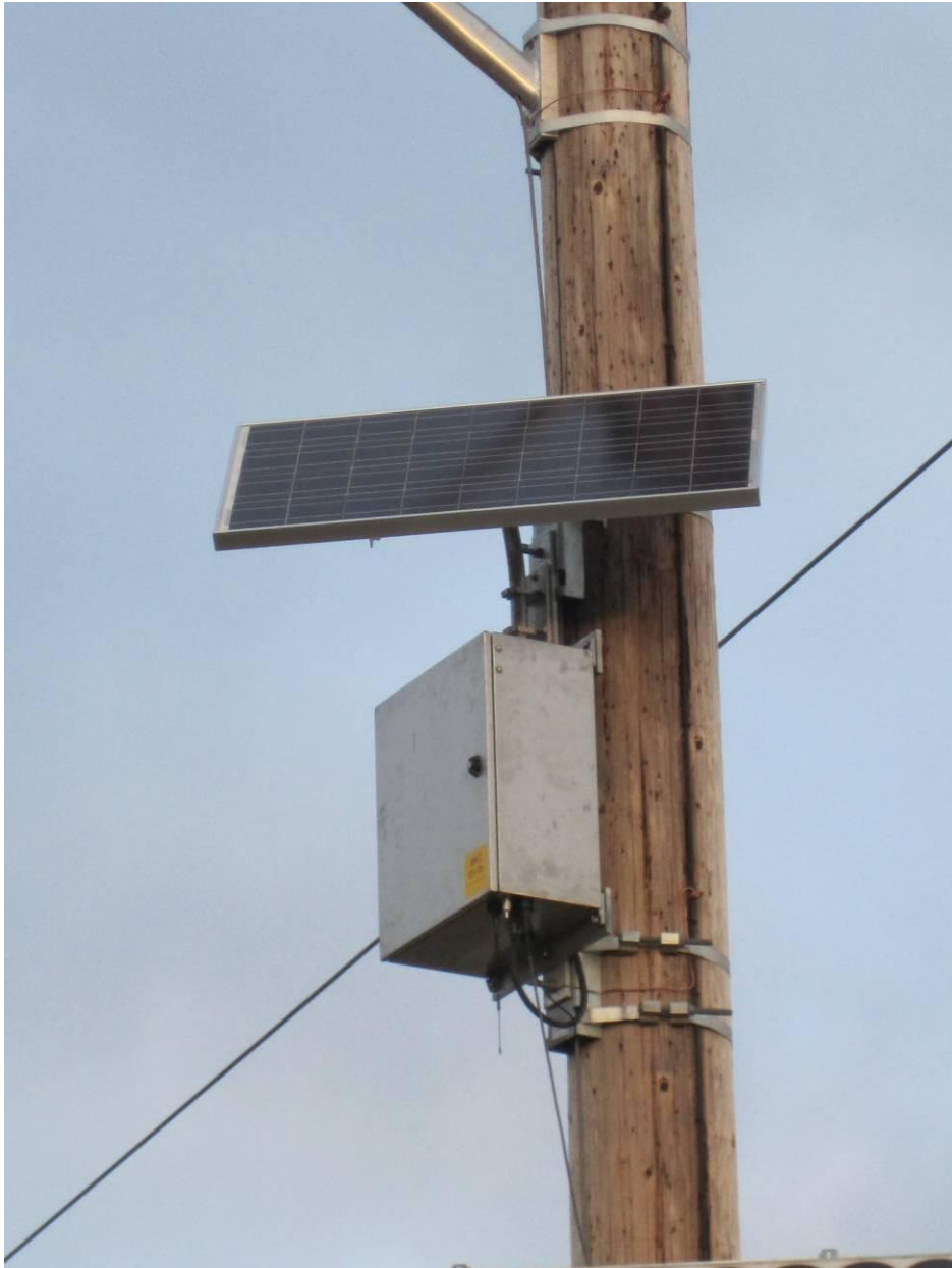
Figure 3-32 Photo of solar System
