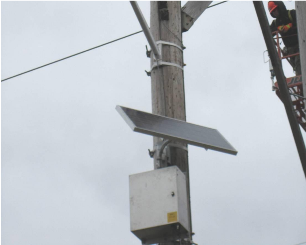
Figure 4-60 EPRI Sensor electronics box and solar panel
