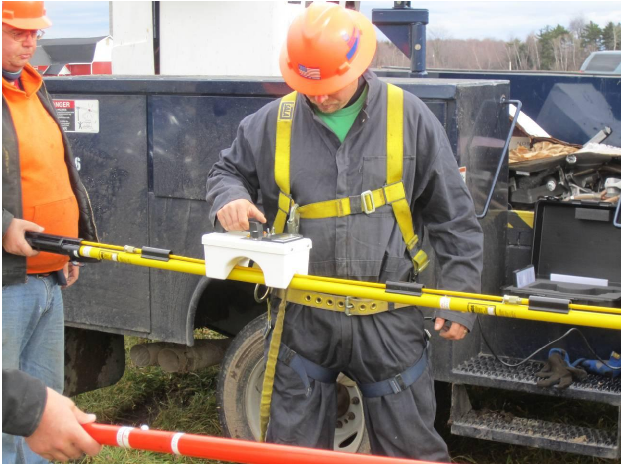
Figure 4-39 Lineman tests hotstick prior to installing the EPRI sensors on the energized 230 kV line
