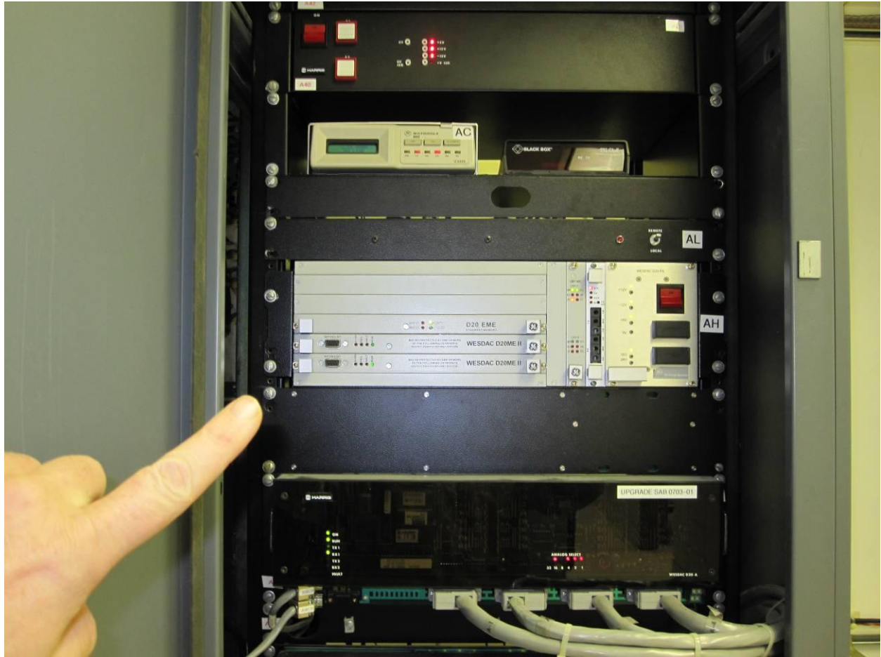
Figure 3-37 RTU at Willis Substation
