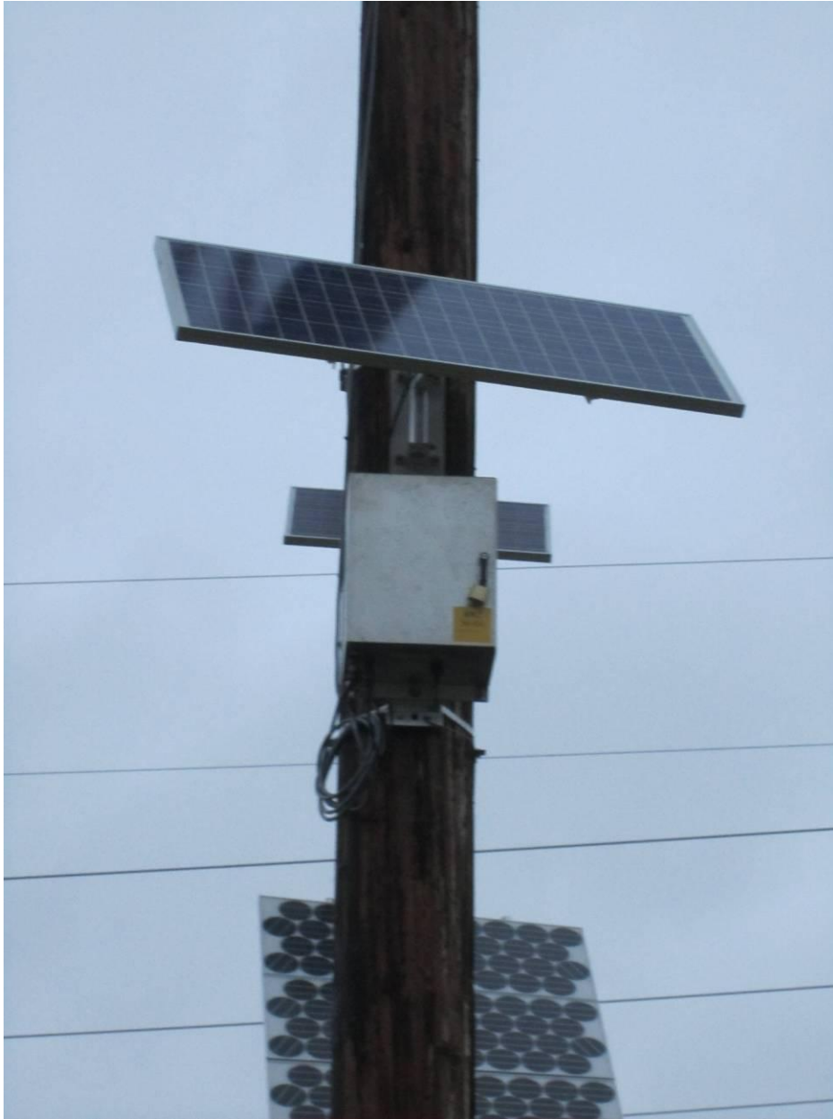
Figure 4-49 Sagometer electronics box and solar panel installed
