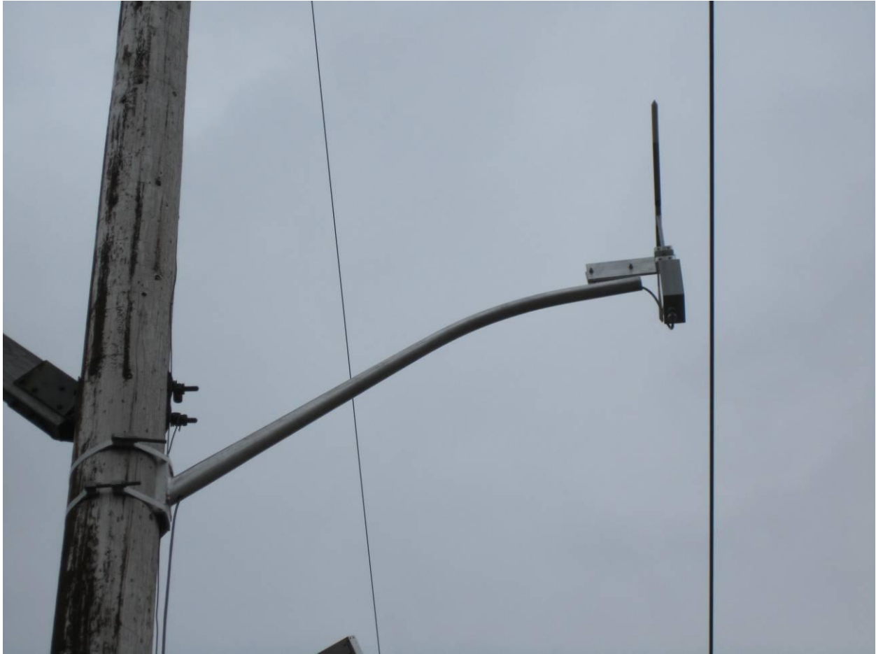
Figure 4-61 ThermalRate sensor and arm installed
