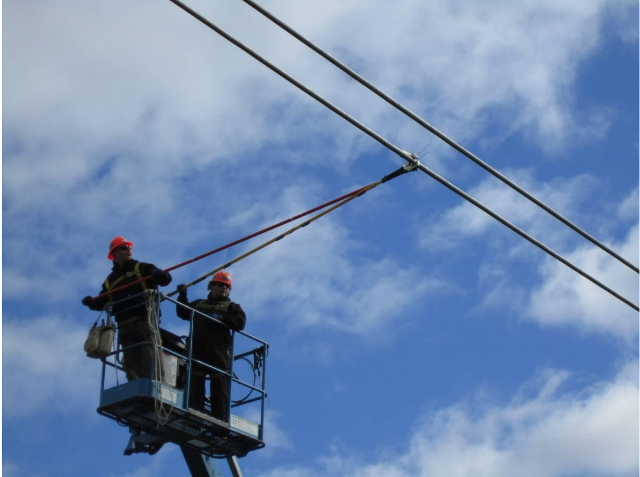
Figure 4-3 The EPRI sensor is being installed on a test line at the Lenox lab
