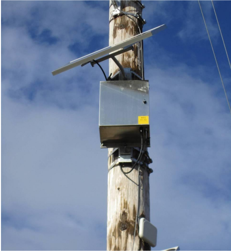
Figure 4-23 EPRI sensor electronics box and solar panel installed
