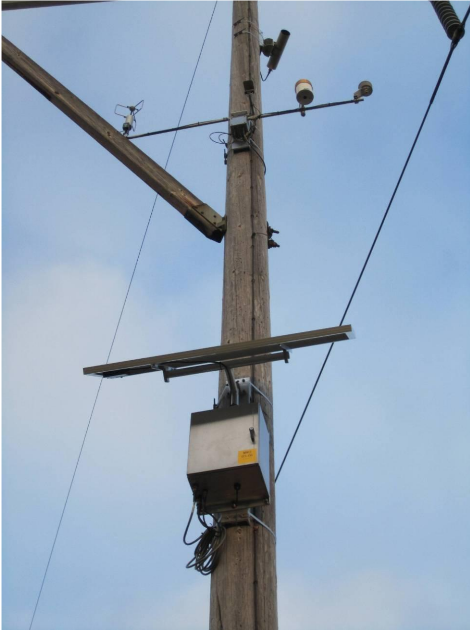
Figure 4-67 Sagometer camera, weather sensors, solar panel and electronics box
