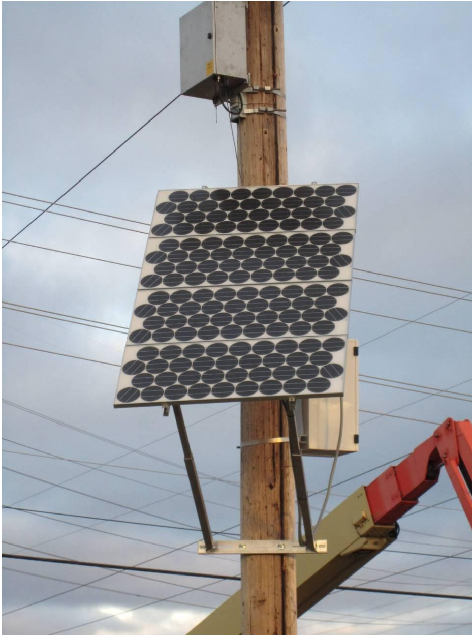
Figure 4-63 ThermalRate solar panel installed
