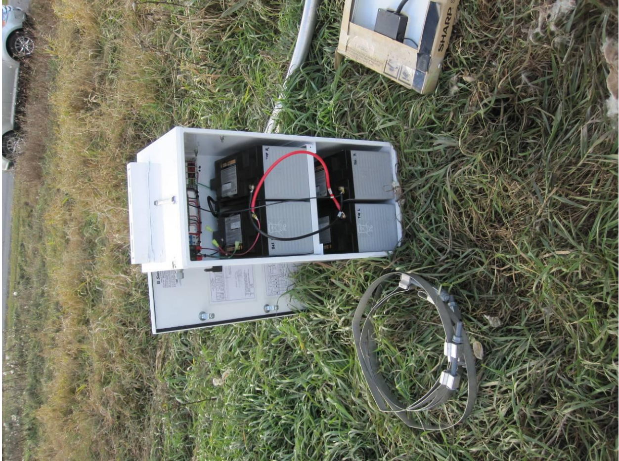
Figure 3-35 Photo of battery and charger
