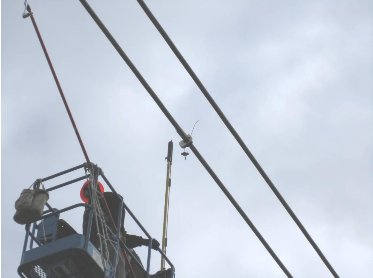
Figure 4-4 Bonding tip becomes stuck during the first install attempt.
