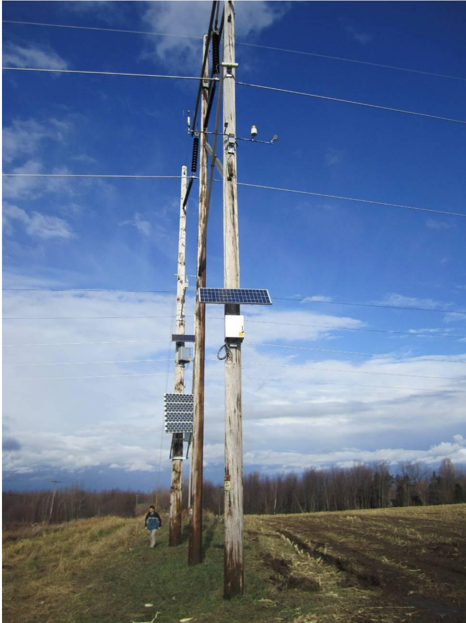
Figure 3-31 Photo of solar System
