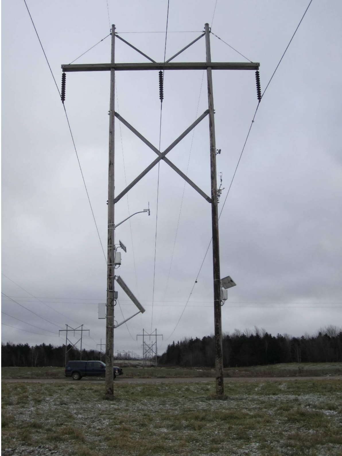
Figure 4-51 Install completed at MW2 - 36/04 - looking back towards Willis Substation in an easterly direction
