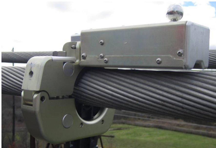
Figure 3-13 EPRI sensor mounted to the conductor.
