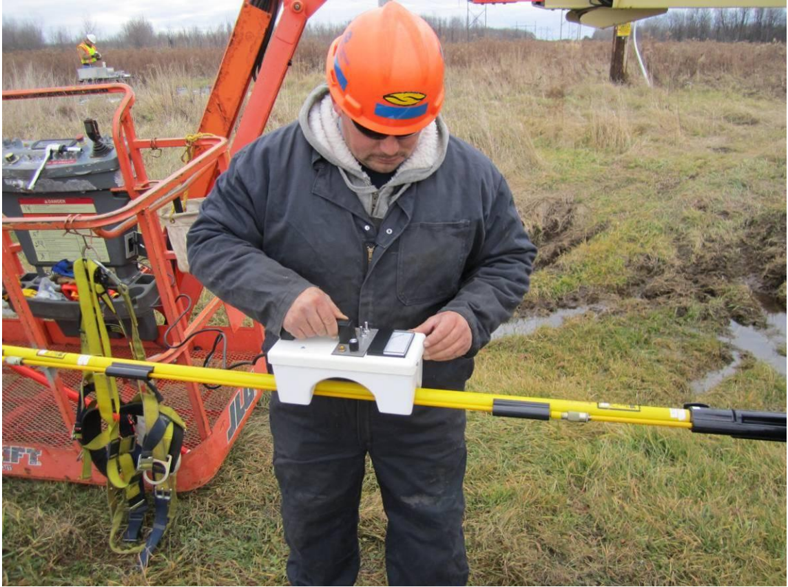
Figure 4-58 Lineman tests hotstick prior to installing the EPRI sensors on the energized 230 kV line
