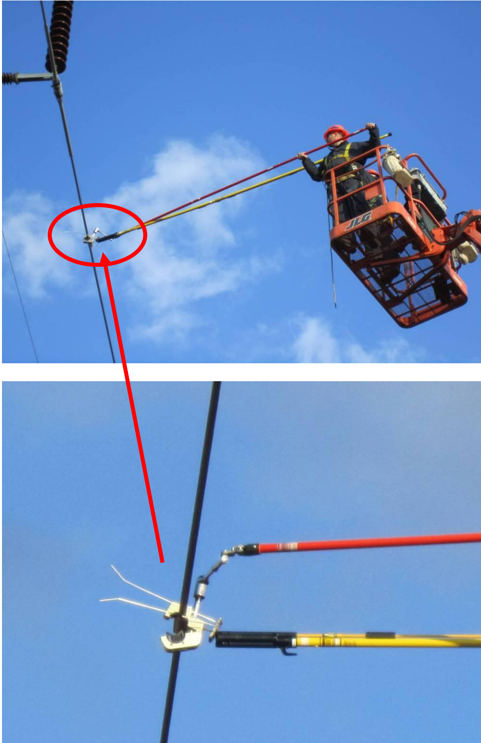
Figure 4-21 EPRI Sensor being installed
