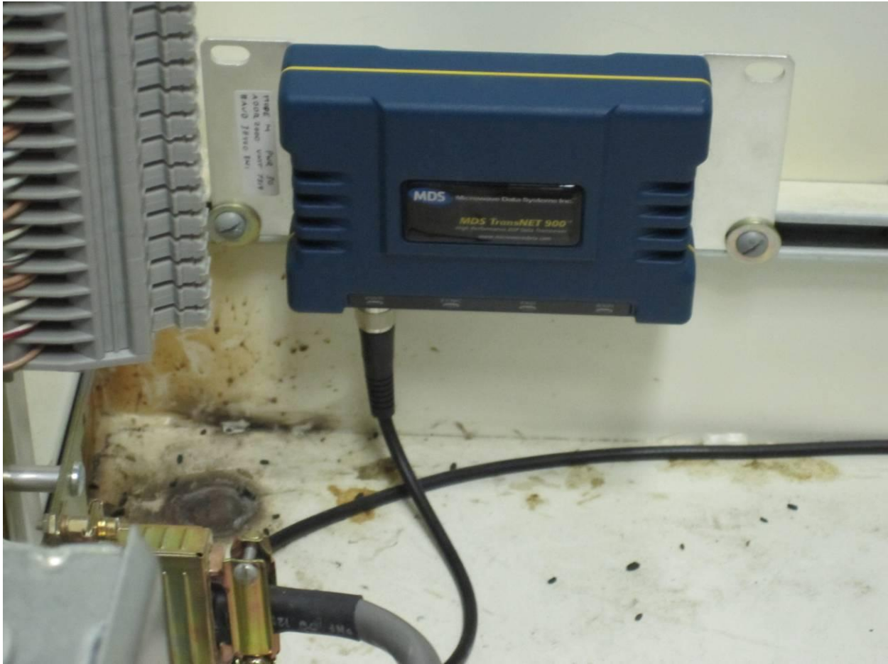
Figure 3-36 Radio communication link (MDS TransNet 900) for ThermalRate system
