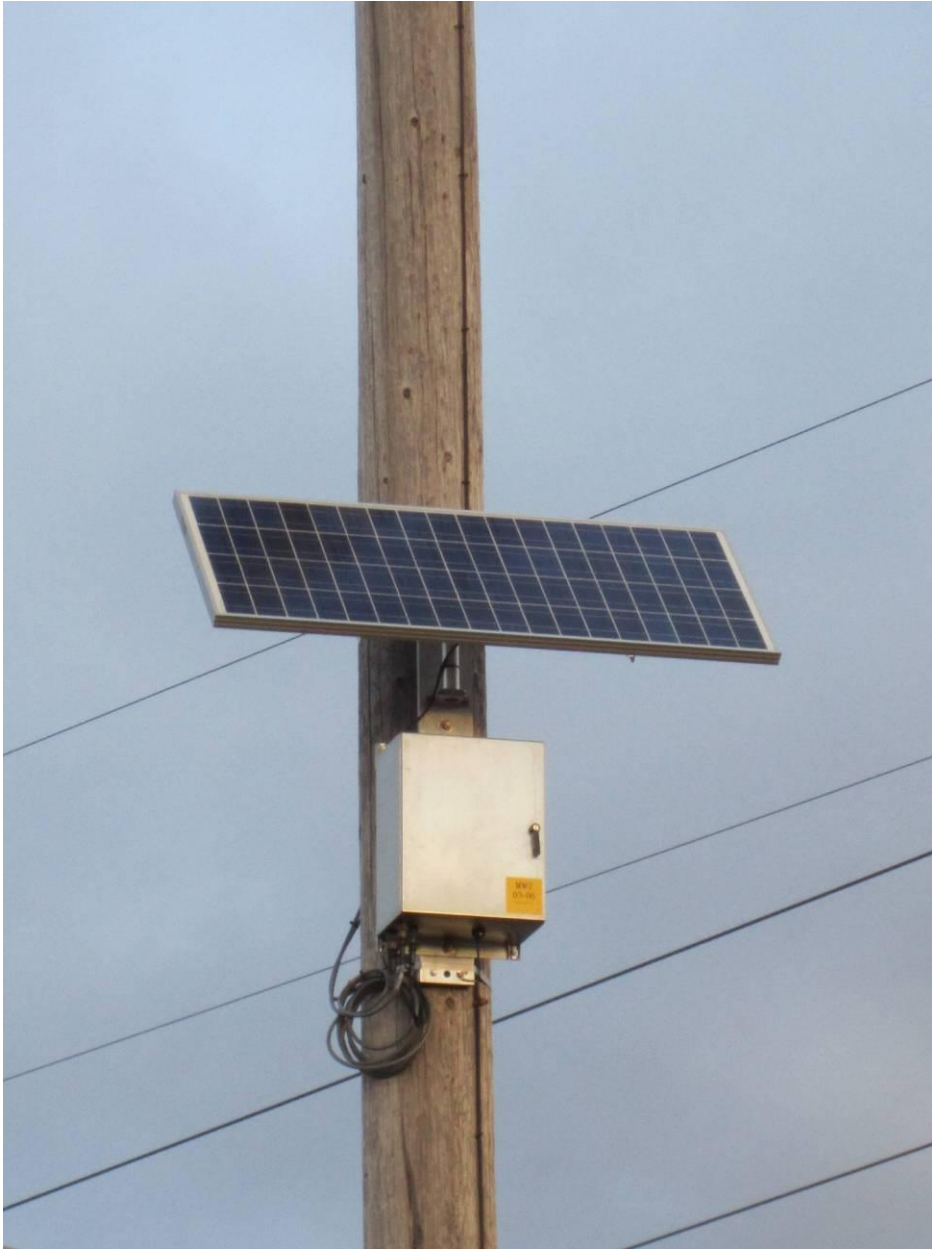
Figure 4-66 Sagometer solar panel and electronics box
