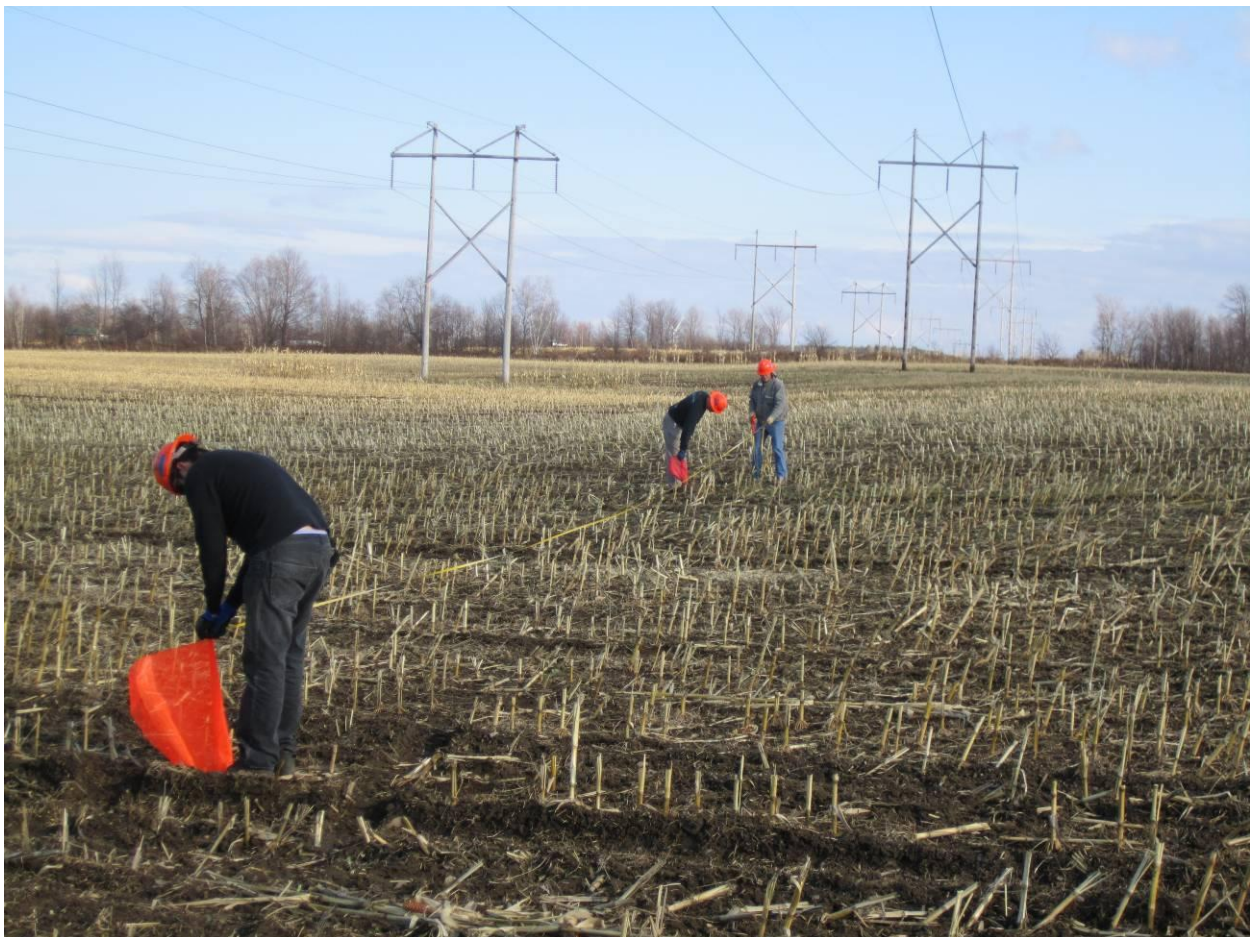
Figure 4-17 Locations were marked under the line for the sagometer target and EPRI sensors
