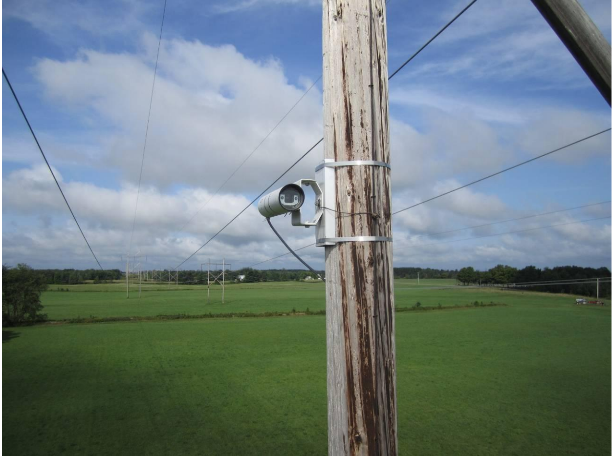
Figure 3-12 Camera unit installed showing the front of the camera. The laser target illumination is mounted inside the camera unit.
