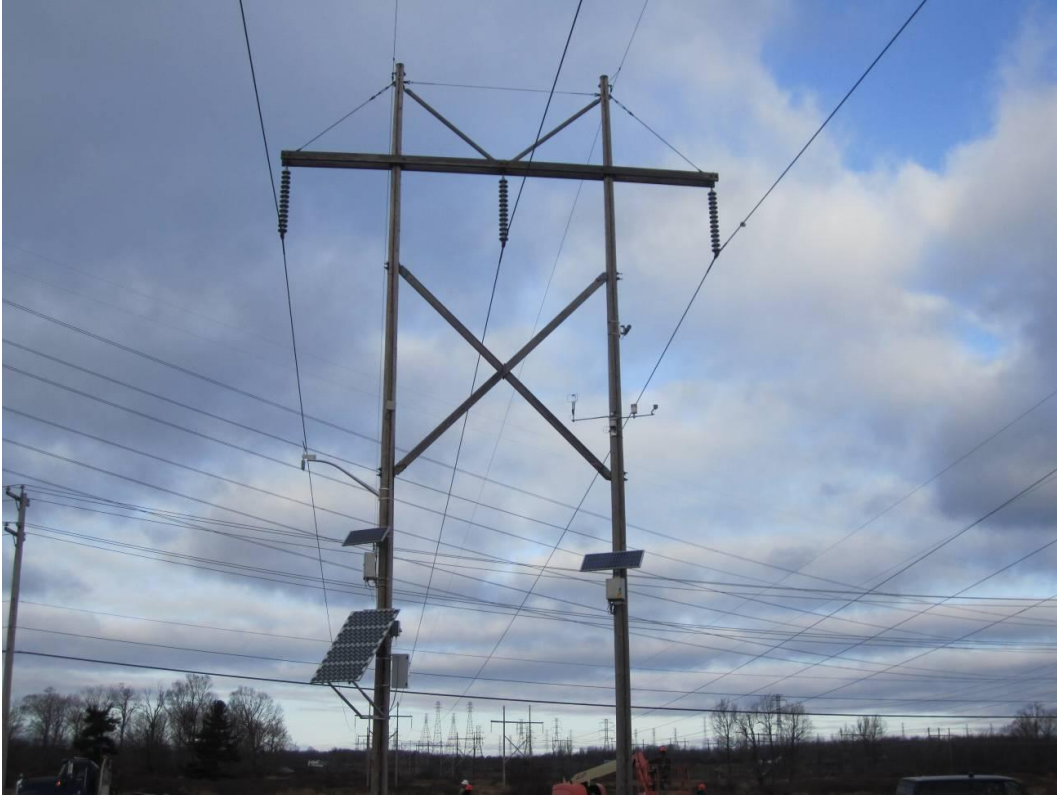
Figure 4-69 MW2 03/06 Completed looking towards Moses Substation
