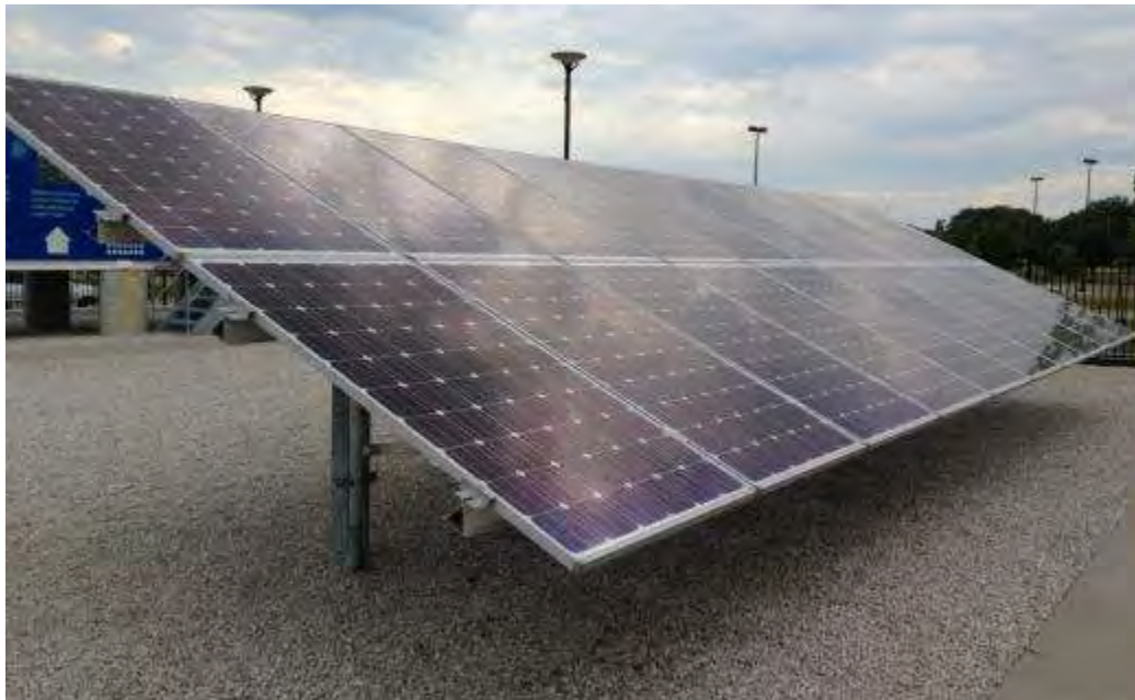
Figure 3-26: 5 kW Photovoltaic Array at SmartGrid Innovation Park
