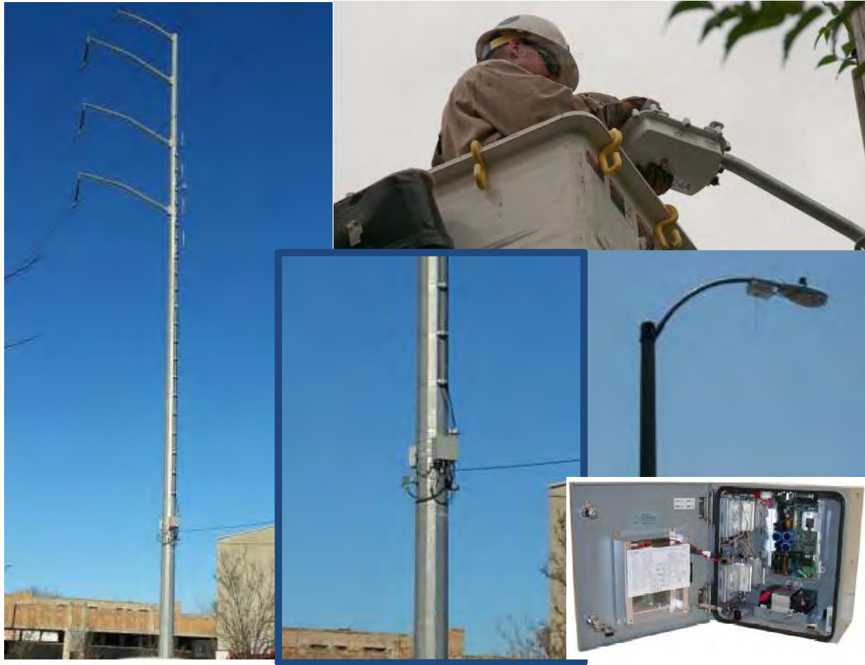
Figure 2-21 Installed AMI FAN Infrastructure
