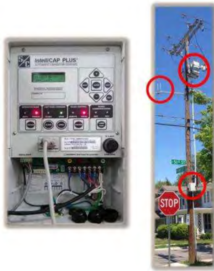
Figure 2-55: Typical Capacitor Bank Installation
