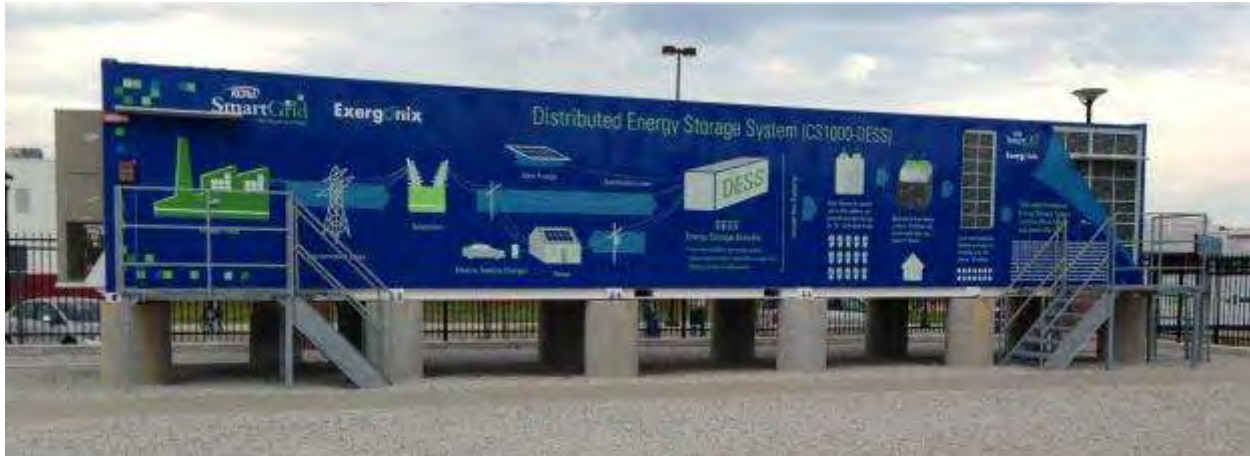
Figure 3-25: Battery Energy Storage System (BESS) at SmartGrid Innovation Park
