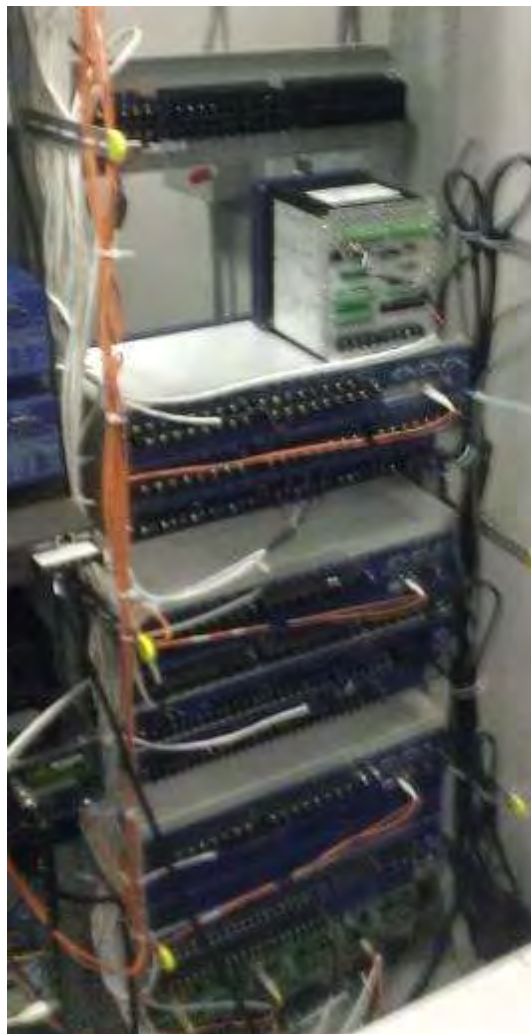
Figure 2-47: GOOSE Lab Testing Rack Setup
