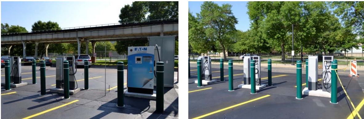
Figure 3.14: Electric vehicle charging stations
