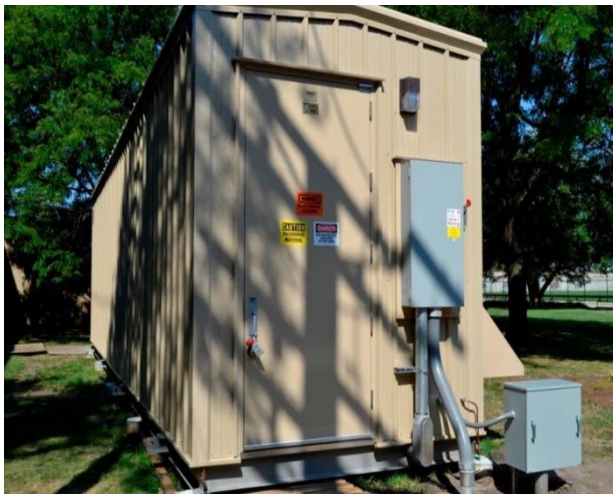
Figure 3.12: IIT Microgrid flow battery
