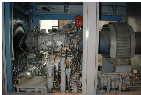
Figure 3.11: The interior of the natural-gas turbine generator
