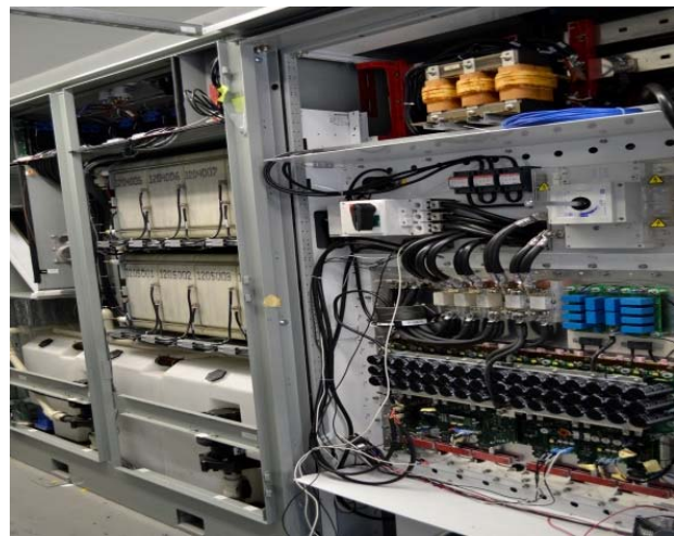
Figure 3.13: Battery storage unit and inverter
