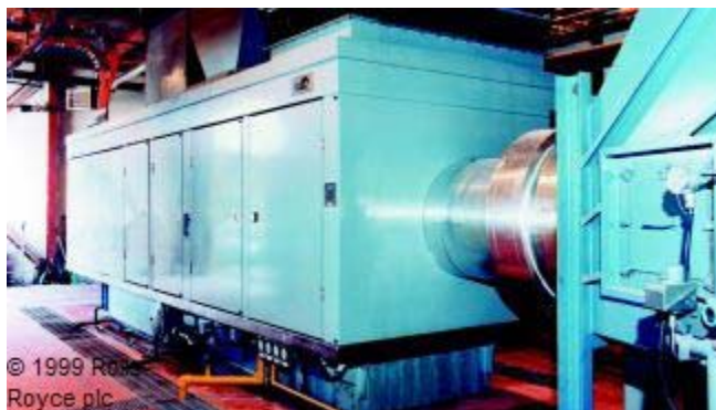
Figure 3.10: The exterior of the natural-gas turbine generator
