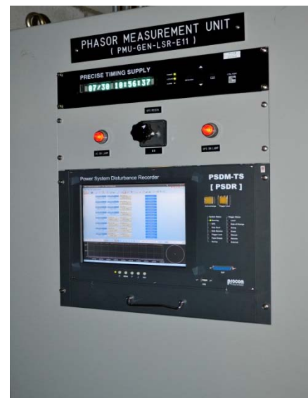
Figure 3.15: PMU at North Substation
