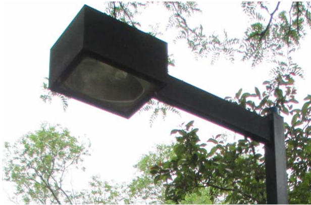
Old High Pressure Sodium (HPS) Lamps
