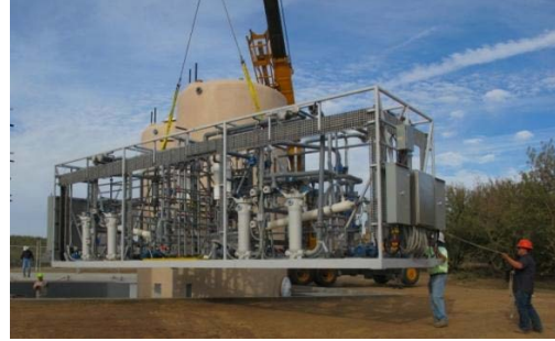
Figure 4 - Skid-mounted Hydraulic Plant Module
