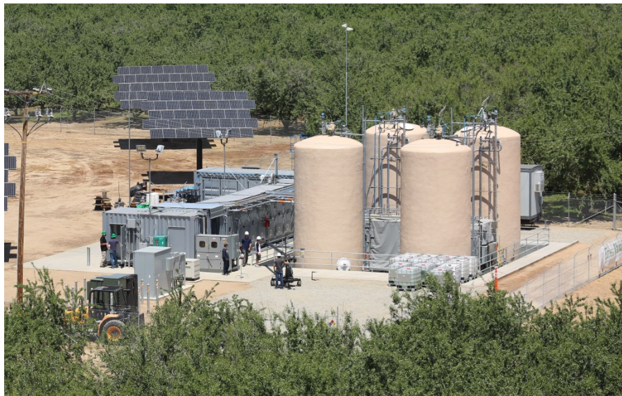
Figure 1 - EnerVault installation in Turlock, CA.
