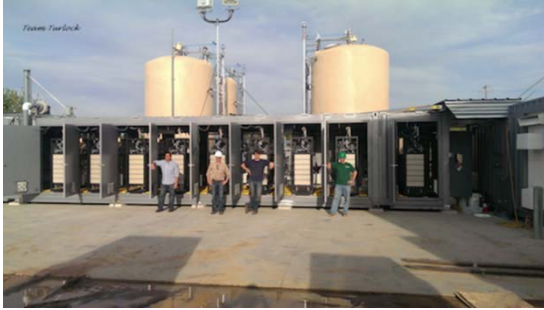
Figure 3 - 30 kW DC cascades installed (9 in total)
