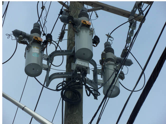
DTE is deploying triple single reclosers on the overhead circuits to isolate faults and remotely monitor current and voltage. The devices allow system supervisors increased ability to perform remote circuit switching to reduce outage time.
