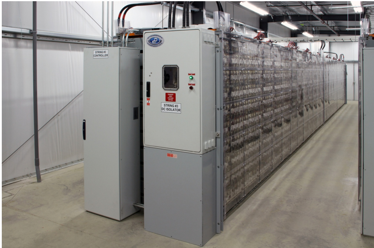
Figure 4. Three strings of batteries installed in the building.
