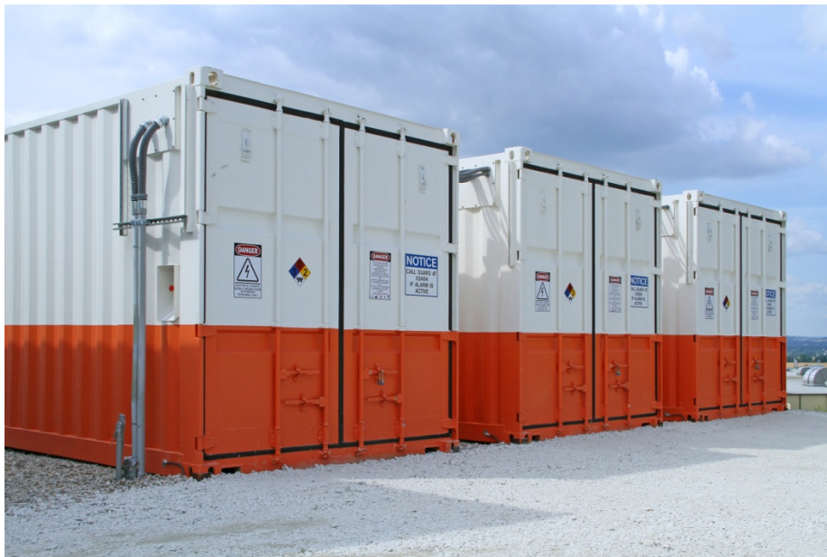
Figure 5. One string of Containerized UltraBattery® System (CUBS)
