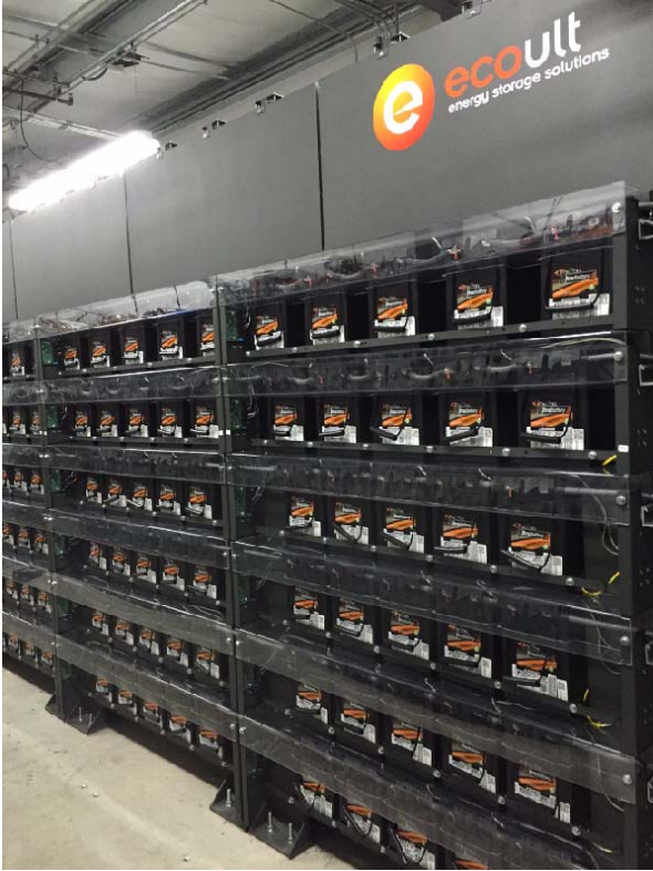
Figure 6. Storage Block #3 utilizing new rack design and new battery design.
