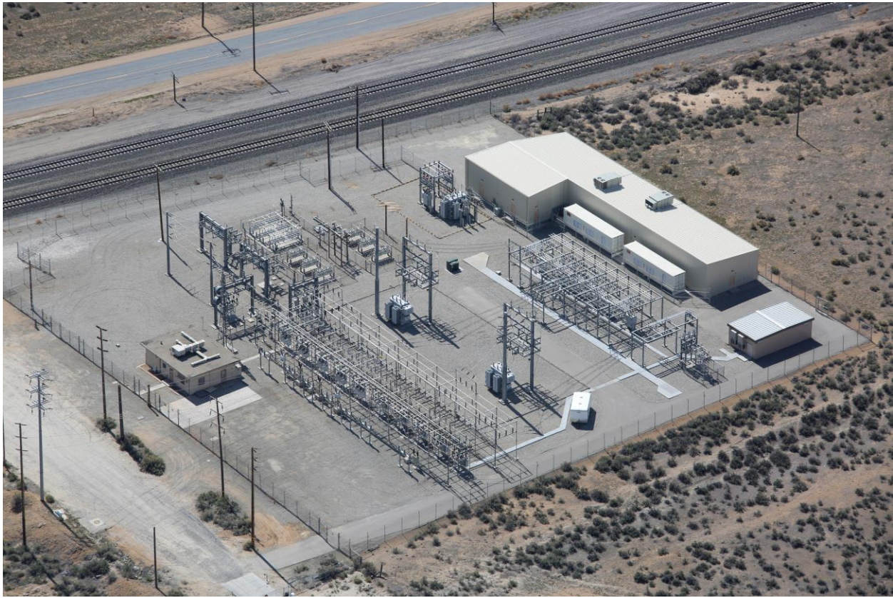
Figure 3-1 Monolith Substation and BESS Facility
