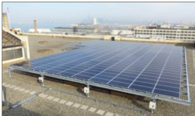
Figure A-65. 100 kW Solar PV Array at BAT
