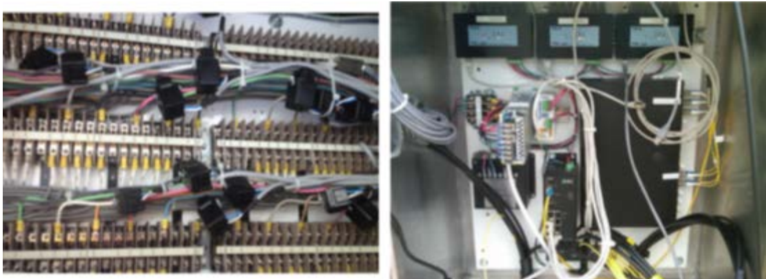
Figure A-75. Breaker Monitor: Sensors (left), Samplers, and Switches (right)
