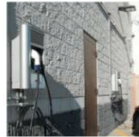
EV Charging Level 2 and Level 3
