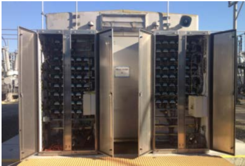
Figure A-69. In-Service Deployment at the Farragut Substation
