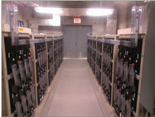
Figure A-64. 720 kWh Battery Installation at BAT
