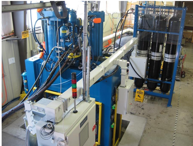
Figure 7: 40 kW Pilot unit at the original Lebanon, NH location, showing cylinders and air storage vessels (back right)
