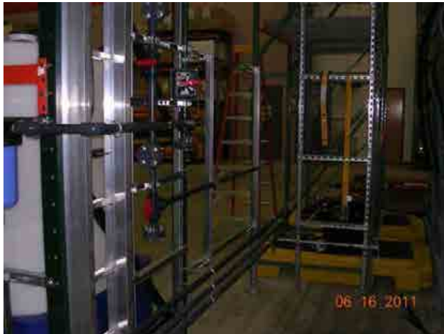
Figure 22 Side View of Positive Electrolyte Sump and Pumps.
