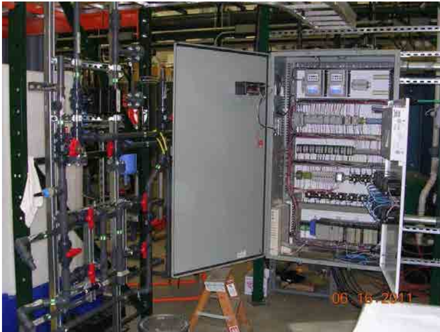
Figure 23 Electrical Control Panel and Right Side of Negative Sump.
