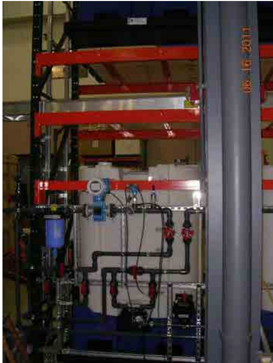
Figure 21 Rear of Negative Electrolyte Sump.
