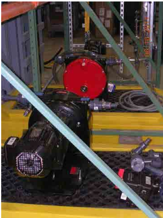
Figure 24 Peristaltic Pumps on Spill Containment Skids.
