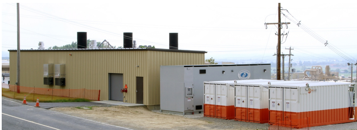
Figure 1. Frequency regulation site at East Penn's facility in Lyon Station, PA.
