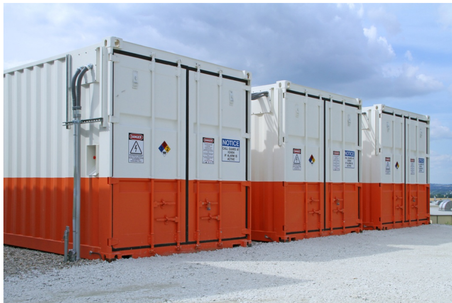
Figure 4. One string of Containerized UltraBattery System (CUBS)
