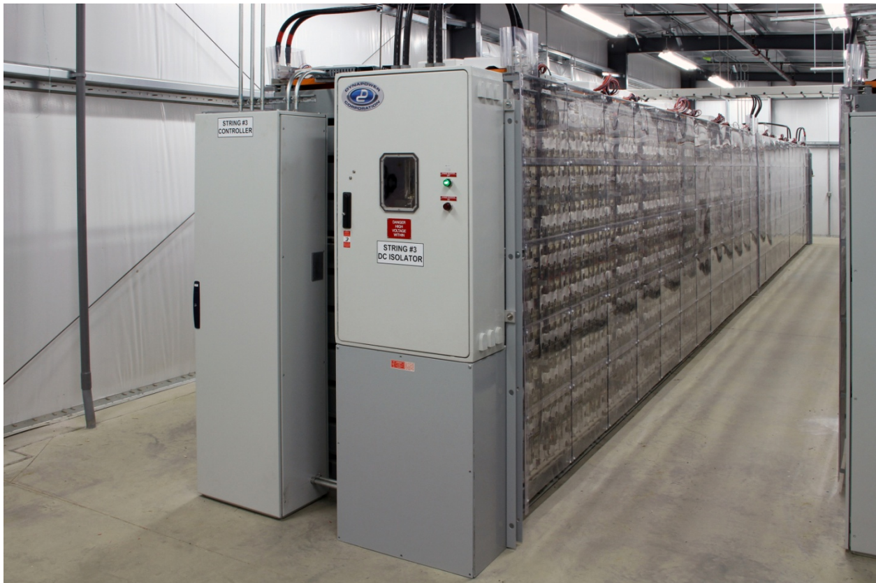
Figure 3. Three strings of batteries installed in the building.
