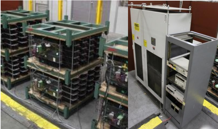
Figure 5 - DOE Test System at Aquion Headquarters
