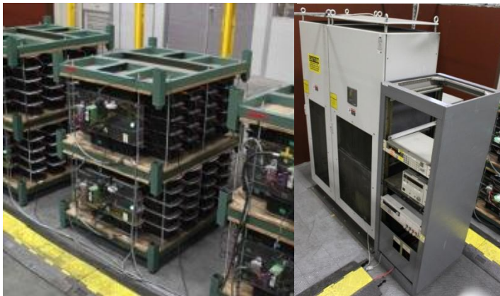
Figure 17 - High Voltage test system battery stacks and inverter setup
